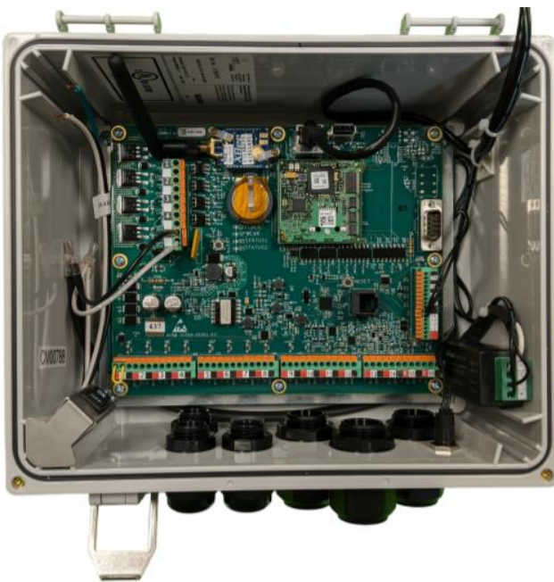
CMM (Control and Monitoring Master)
