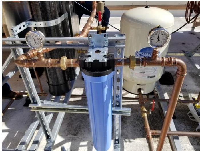
Figure 6. Filter Assembly Installed with water pressure gauges
