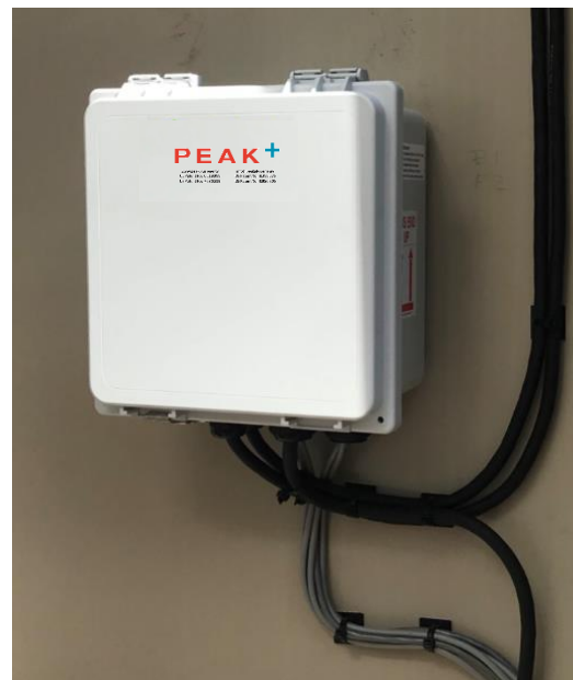
Figure 27. (Above) Master Controller as mounted
