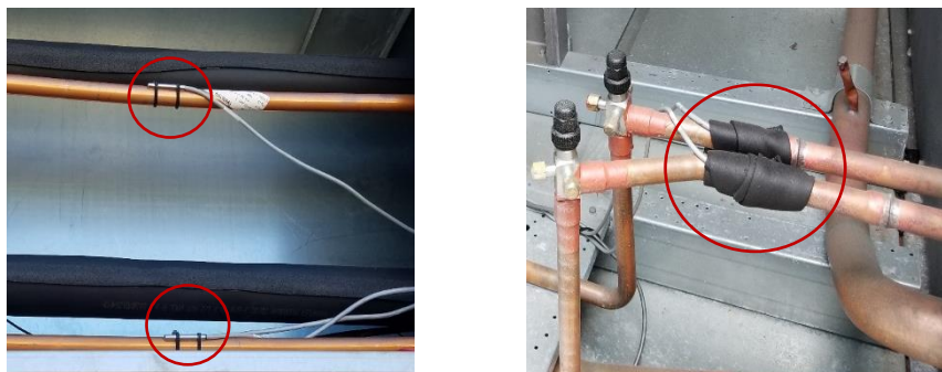
Figure 43. Liquid line temperature sensor, zip-tied before insulating
