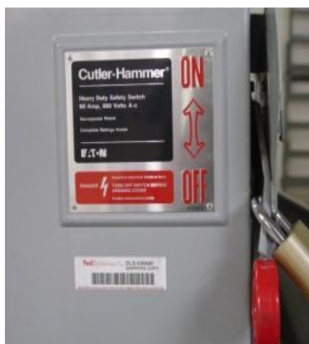
Figure 25. Locked out/tagged out disconnect
