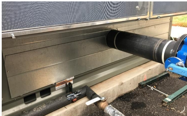
Figure 55. Sheet metal used to seal off openings surrounding a chilled water pipe
