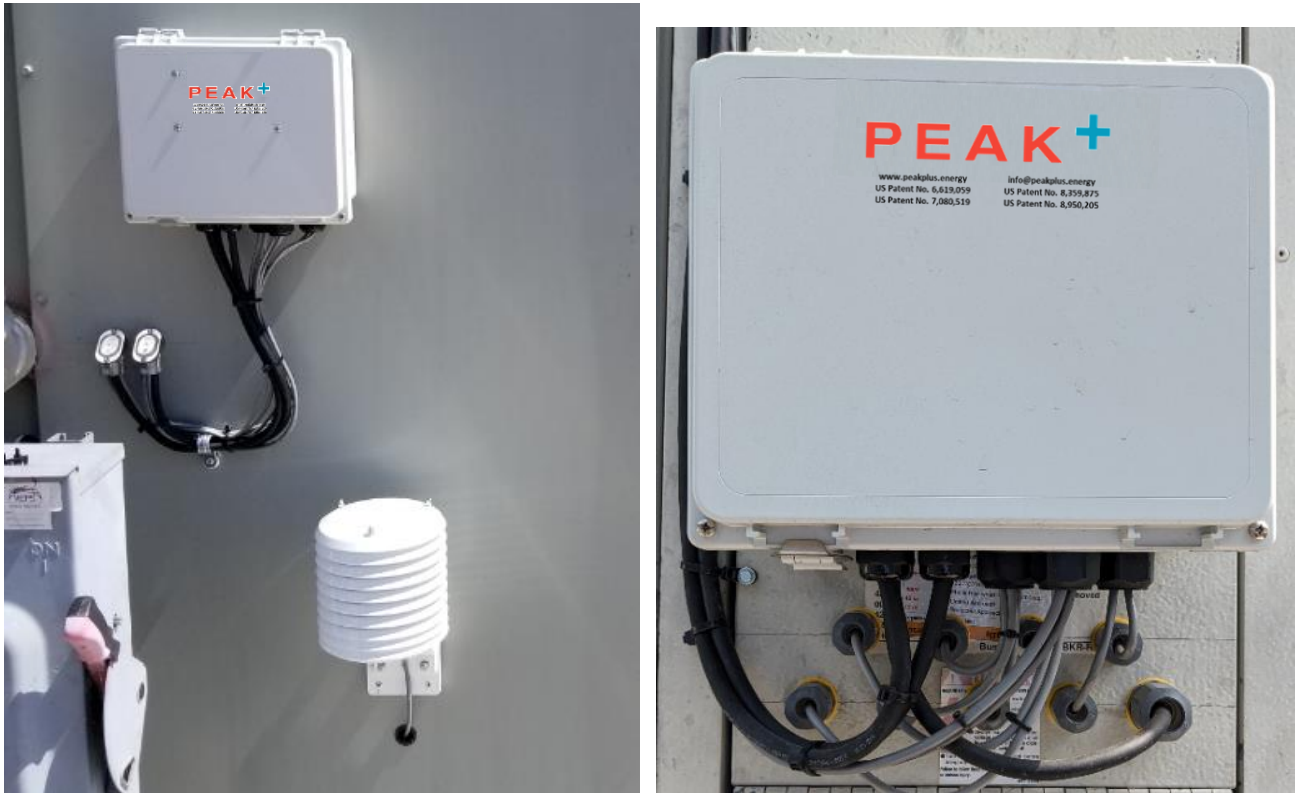
Figure 36. Master controller (CMM) mounted with wiring connected
