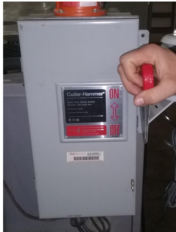
Figure 42. Restoring power to disconnect
